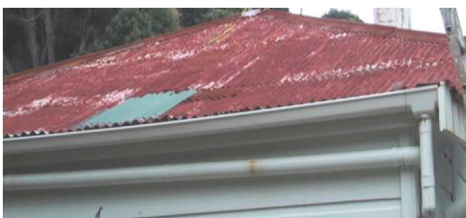
Do not restore any roof material type where the product is beyond its useful life
